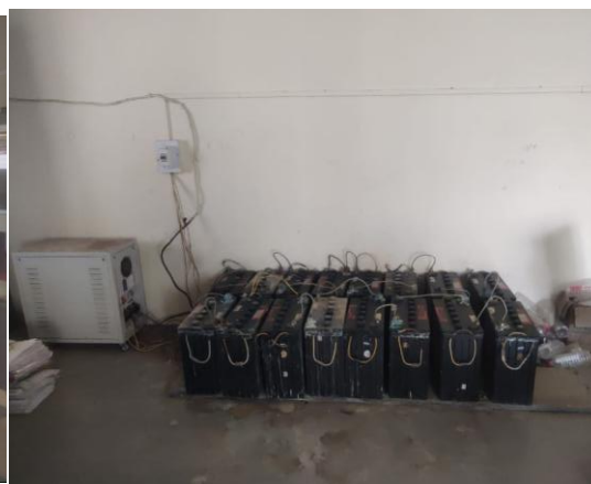
b. Battery Backup
